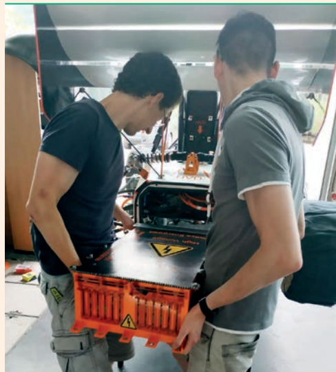
■ Fig. 2: Installation of the battery in the race car (Photo: © Elefant Racing).
